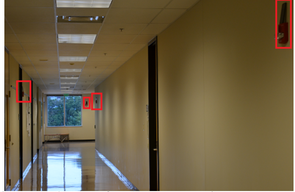
Figure 7: A part of the testbed showing smartphones (hanging near the fire alarms) that served as gateways.
