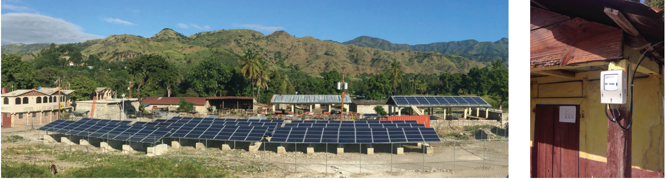
Figure 2: Solar PV array with battery and diesel generation (left) and Sparkmeter hardware (right)
