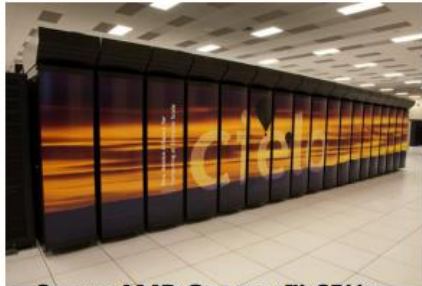
Cielo at Los Alamos National Lab
