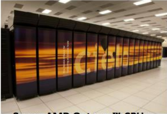
Cielo at Los Alamos National Lab
